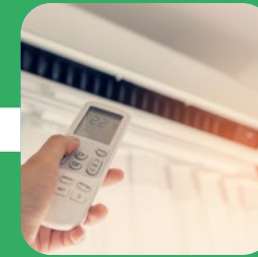
Variable Refrigerant Volume Cooling System
